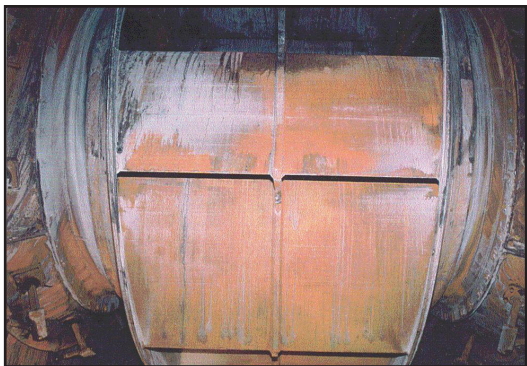
Fig. 1. Overall view of Induced Draft Fan.
