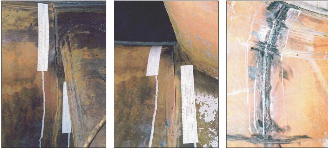
Fig. 3. Photographs of severe fan cracking and subsequent weld repair.
